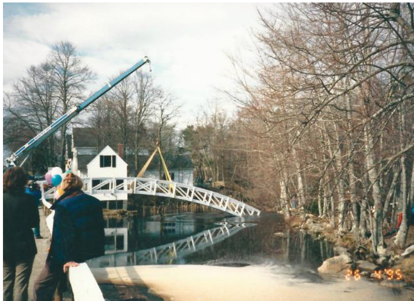
A replacement bridge, built with pressure-treated lumber, is installed in 1995. Mount Desert Island Historical Society
